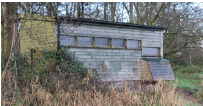
Bird hide exterior showing lowered viewing hatch with knee space below, Moyola Nature Reserve
