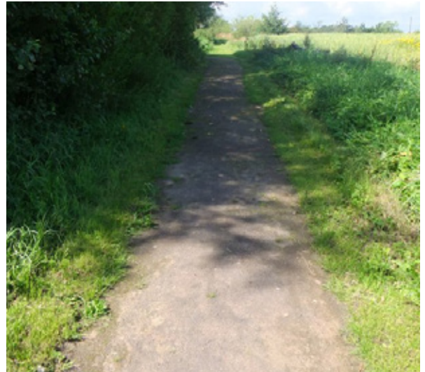
Well-compacted, firm whin dust ground surface used on level terrain, Portmore Lough Nature Reserve (Image courtesy of RSPB)
